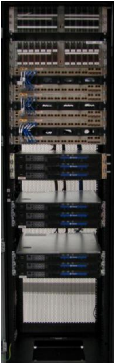
Figure 3: Tekelec T1200 Application Cabinet
