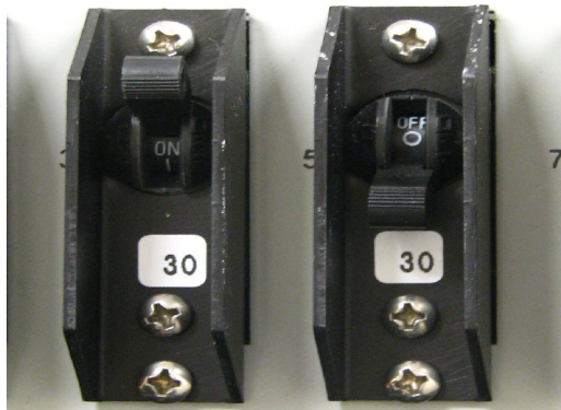
Figure 8: Locate Failed Breaker
