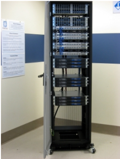
Figure 44: Example of T1200 cabinet with Pre-cabled Components shows the same T1200 application cabinet with a view of the pre-cabled components.
