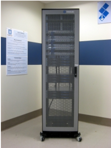
Figure 43: T1200 cabinet with Pre-installed Components shows the same T1200 cabinet with a view of the pre-installed components.
