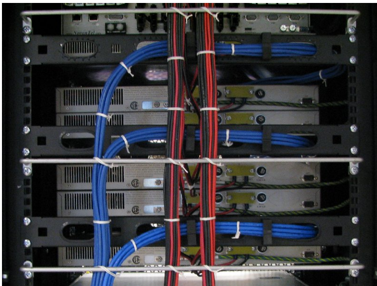
Figure 48: T1200 Application Server Cabling
