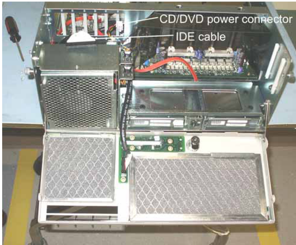
Figure 78: Removable Media Disk Drive Cables (drives removed)
