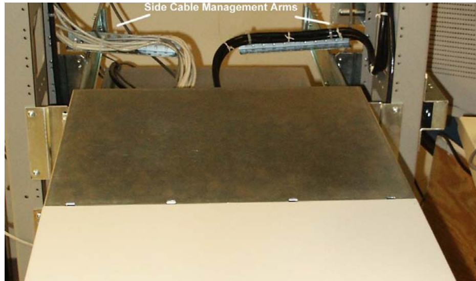
Figure 3-6. T1100 AS with Side Cable Management Arms
