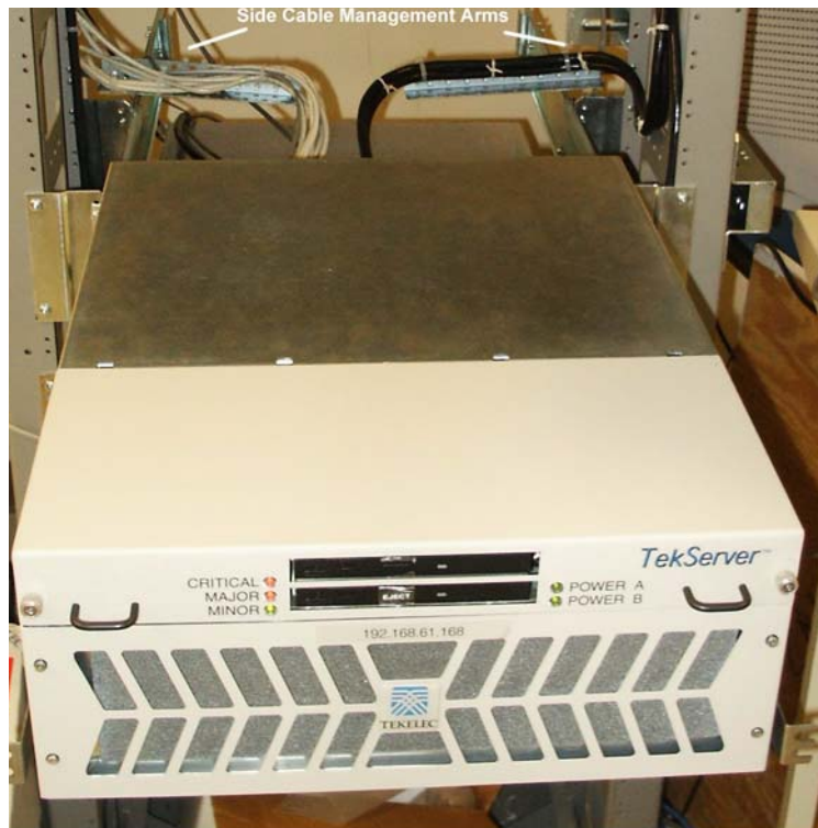
Figure 3-7. T1000 AS with Side Cable Management Arms
