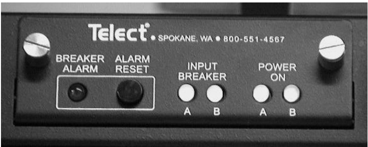
Figure 6-6. Breaker Panel LEDs
