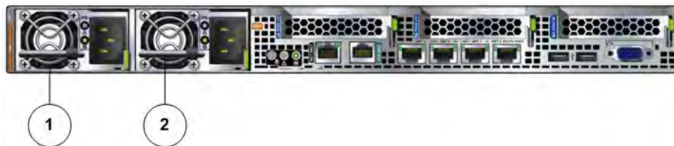
Figure 175: Location of the Pilot power supplies
