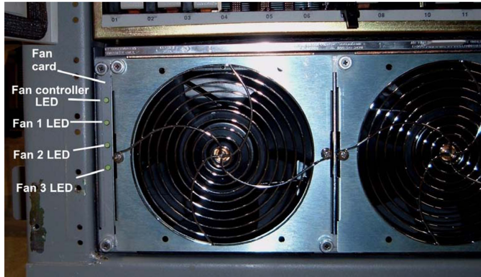
Figure 91: Fan card with LEDs on front of fan assembly
