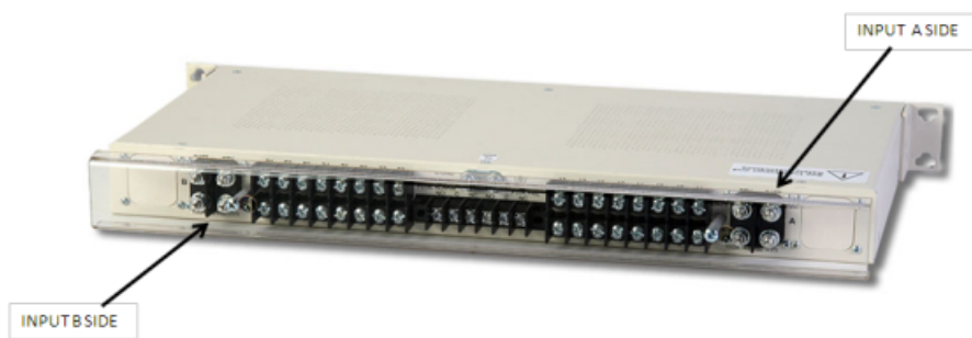
Figure 83: Telect 100A 4/4 fuse panel - rear view
