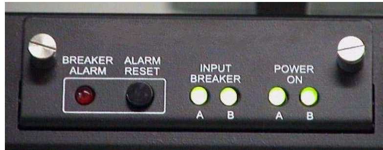
Figure 4-9. Breaker Panel LEDs
