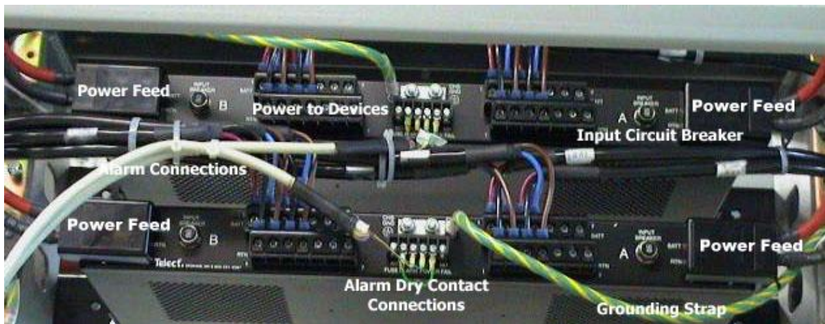
Figure 37: Breaker Panel - Rear Cabling
