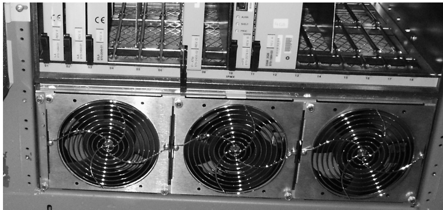
Figure A-26. Fan tray inserted into fan tray bracket in the frame- front view
