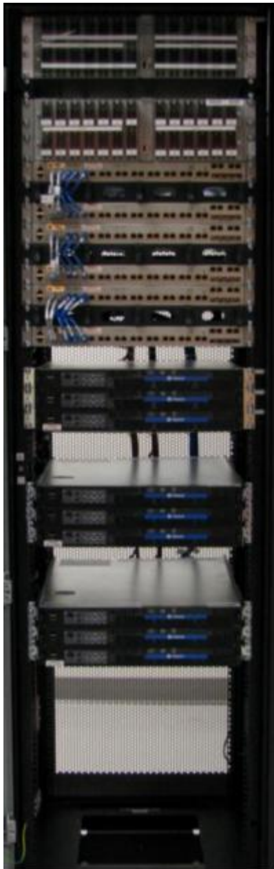
Figure 10: Tekelec T1200 Application Cabinet
