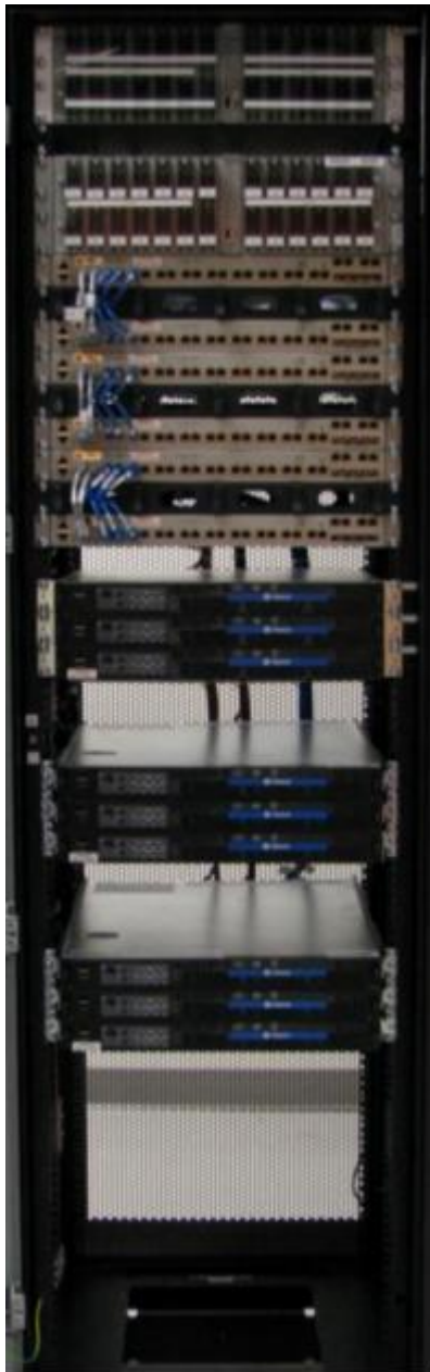
Figure 3: Tekelec T1200 Application Cabinet
