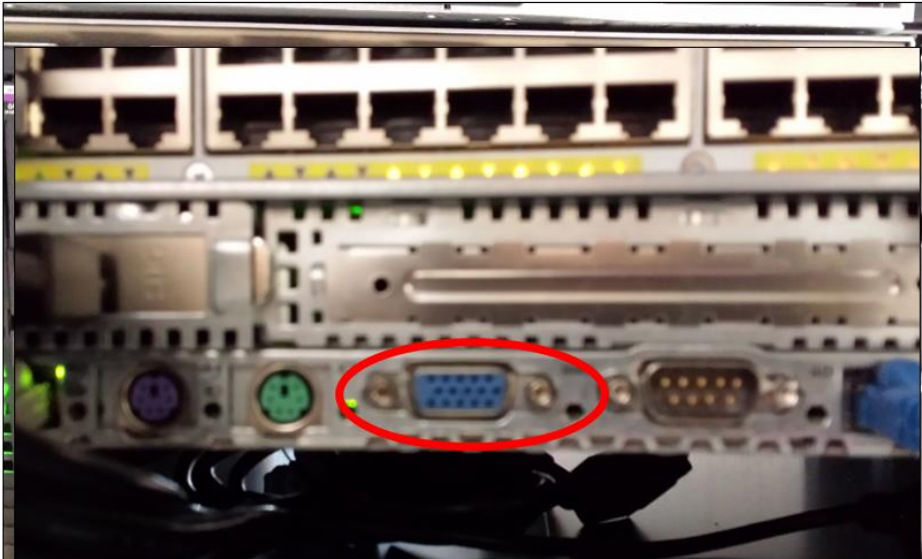
Figure 8. Terminal Video Connection on Rack Mount Server
