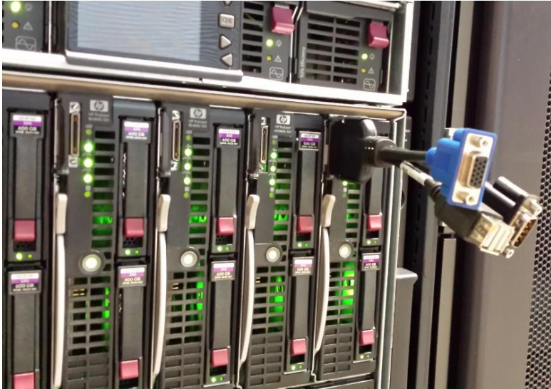
Figure 6. Custom Terminal Key Board Connector Cable Inserted in Local Terminal Connection
