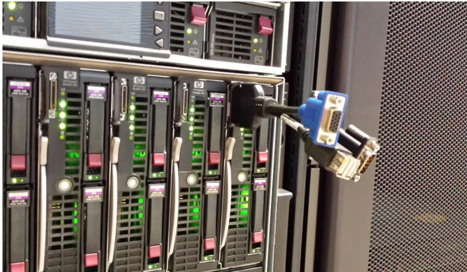
Figure 6 - Picture showing custom cable connection for terminal key board
