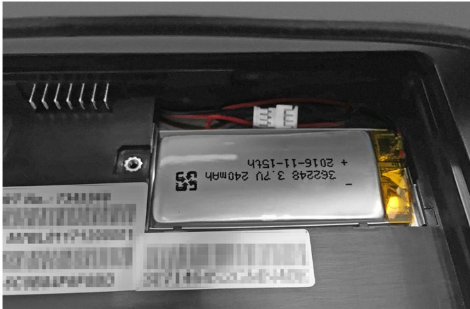
Figure 7-5 The Bridge Battery in the Battery Compartment
