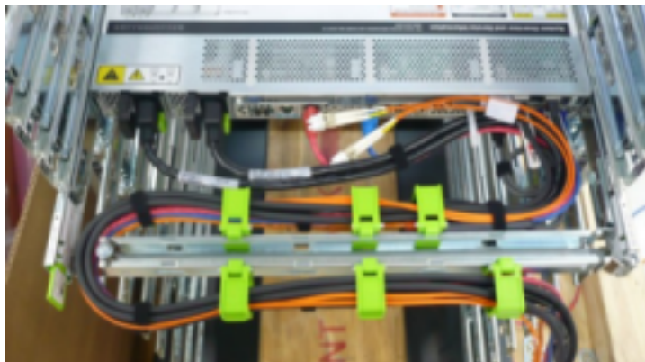
Figure 1-12 InfiniBand or TwinAx Cables Secured with Hook and Loop Straps at Regular Intervals
