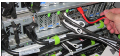
Figure 1-13 Rear of the Server Showing Power and Network Cables
