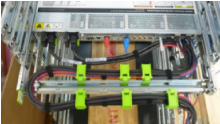
Figure 1-11 InfiniBand or TwinAx Cables Positioned on the CMA
