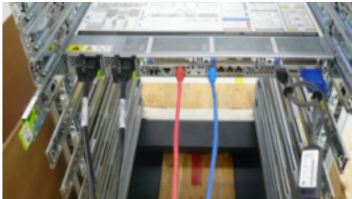
Figure 1-6 Cables at the Rear of the Server
