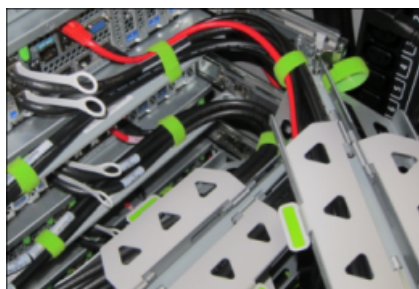
Figure 1-14 Cables Routed Through the CMA and Secured with Hook and Loop Straps
