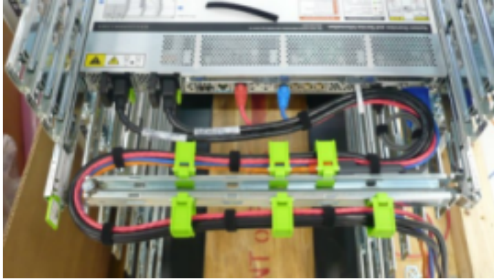
Figure 1-10 Cables Secured with Hook and Loop Straps at Regular Intervals
