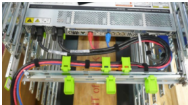
Figure 1-9 Cables Secured under the Cable Clasps
