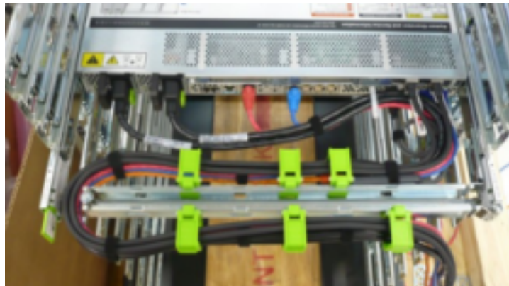
Figure 2-8 RDMA Network Fabric or TwinAx Cables Positioned on the CMA
