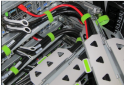
Figure 2-11 Cables Routed Through the CMA and Secured with Hook and Loop Straps
