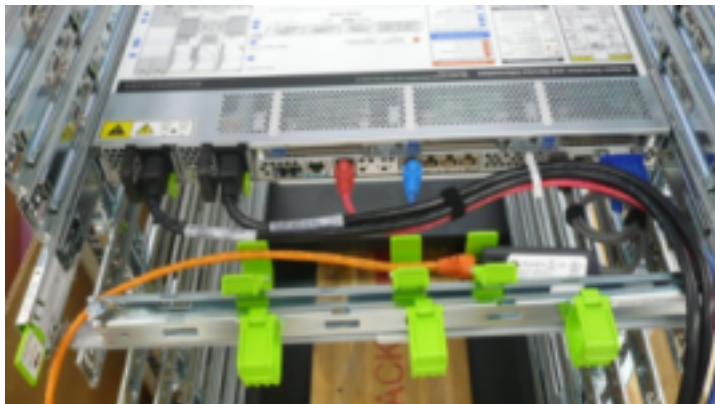
Figure 2-5 Cables Routed Through the Cable Management Arm
