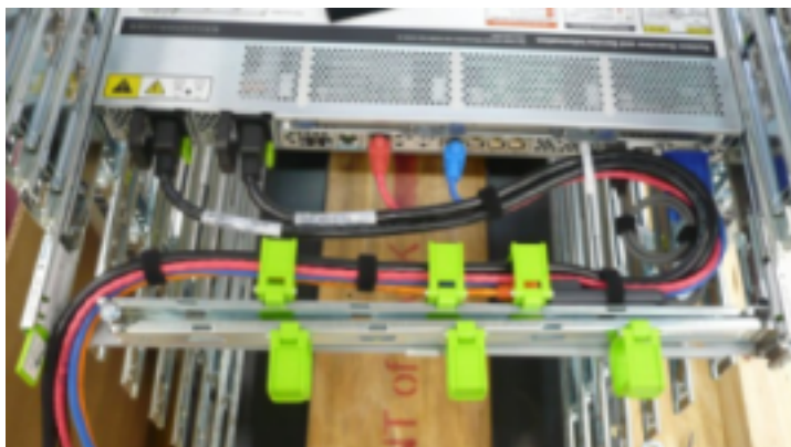
Figure 2-6 Cables Secured under the Cable Clasps
