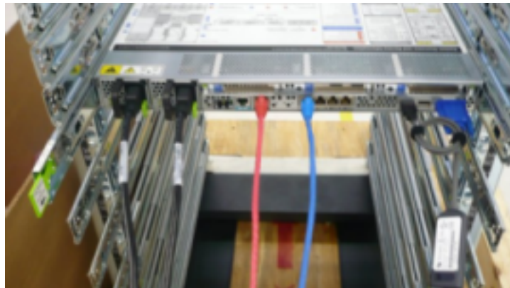
Figure 2-3 Cables at the Rear of the Server
