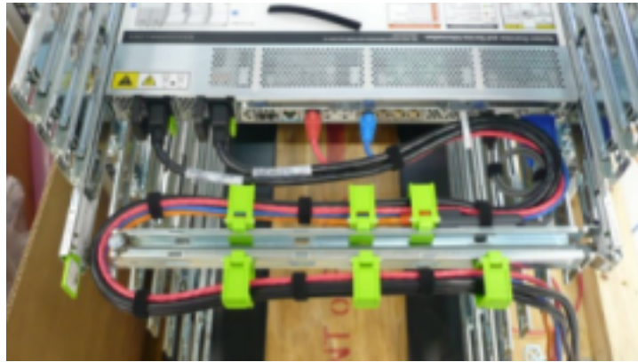
Figure 2-7 Cables Secured with Hook and Loop Straps at Regular Intervals
