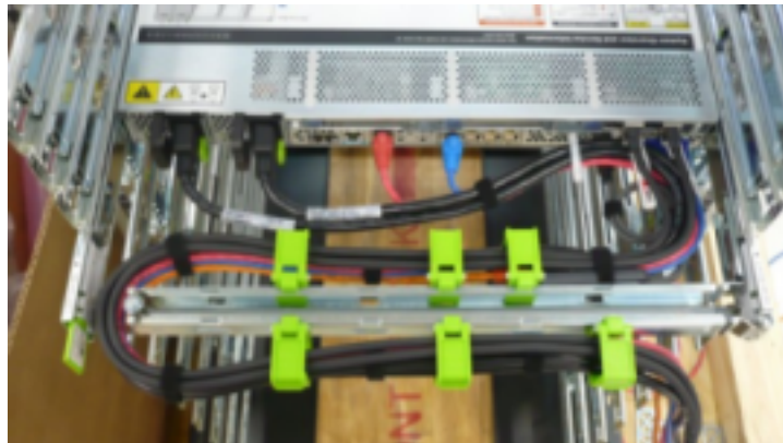
Figure 2-8 RDMA Network Fabric or TwinAx Cables Positioned on the CMA
