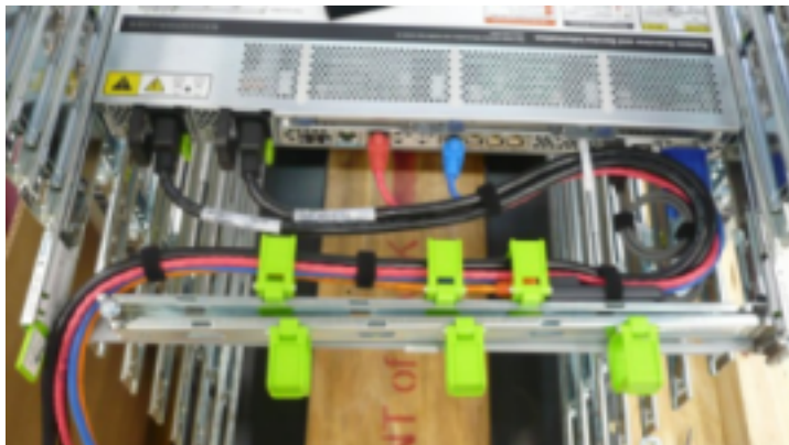
Figure 2-6 Cables Secured under the Cable Clasps
