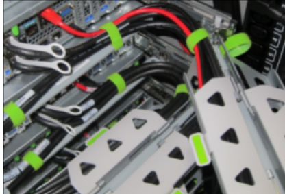
Figure 2-11 Cables Routed Through the CMA and Secured with Hook and Loop Straps
