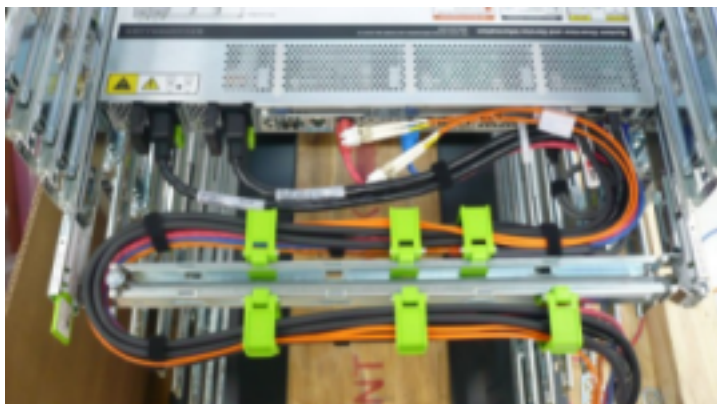
Figure 2-9 RDMA Network Fabric or TwinAx Cables Secured with Hook and Loop Straps at Regular Intervals
