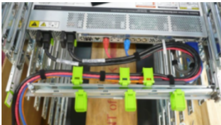
Figure 2-6 Cables Secured under the Cable Clasps
