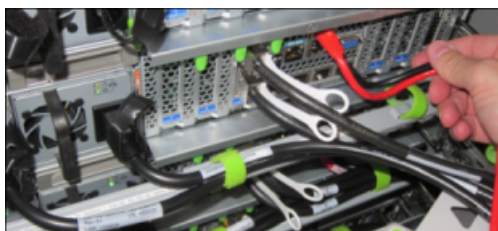
Figure 2-10 Rear of the Server Showing Power and Network Cables
