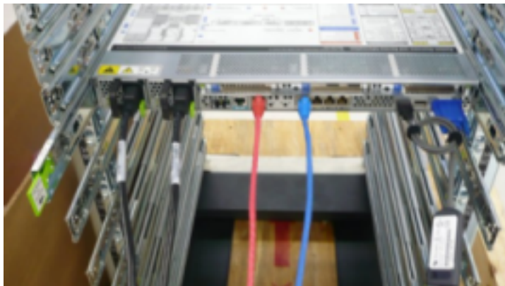
Figure 2-3 Cables at the Rear of the Server
