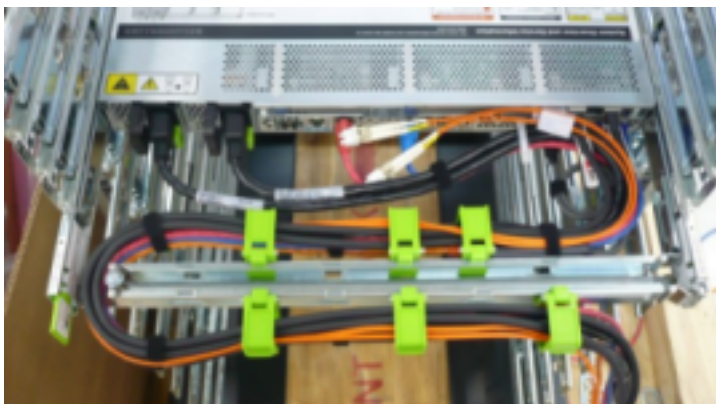
Figure 2-9 RDMA Network Fabric or TwinAx Cables Secured with Hook and Loop Straps at Regular Intervals
