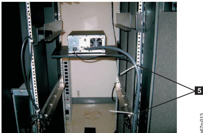
Figure 30. Rear view of shelf with cables attached to rack rails with tie wraps
